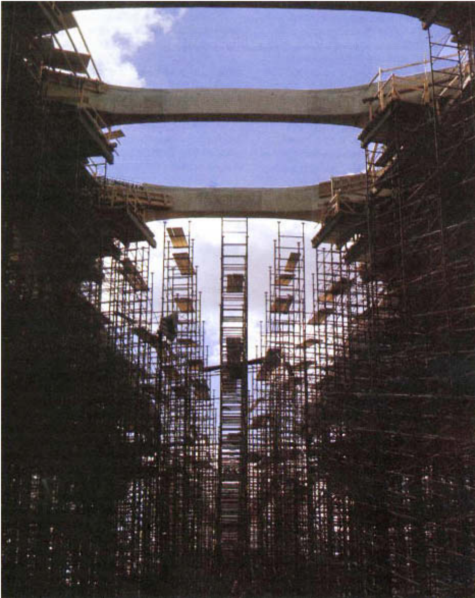
In view of the unstable nature of the ground, the engineers had to change the concept of the scaffolding which was to accommodate the prefabricated voussoirs designed according to the shape of the Olympic Velodrome roof.
